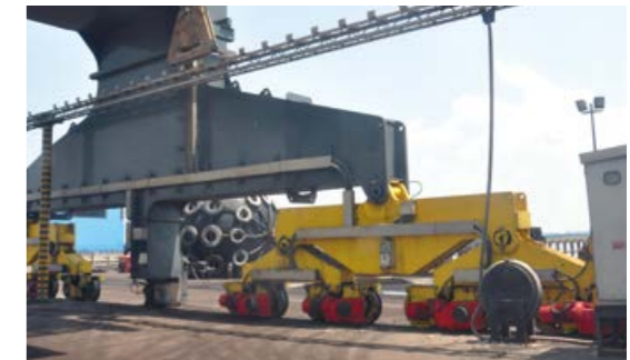
High-level cable guide arrangement allows vehicles to travel under the supply cable.
