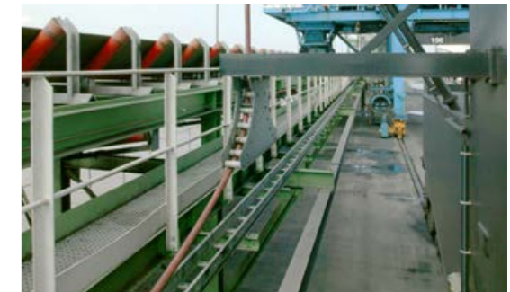
A cable guide alongside the conveyor belt also saves space.
