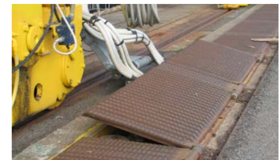
Energy supplied via a busbar of a low-voltage electrical system is also possible.
